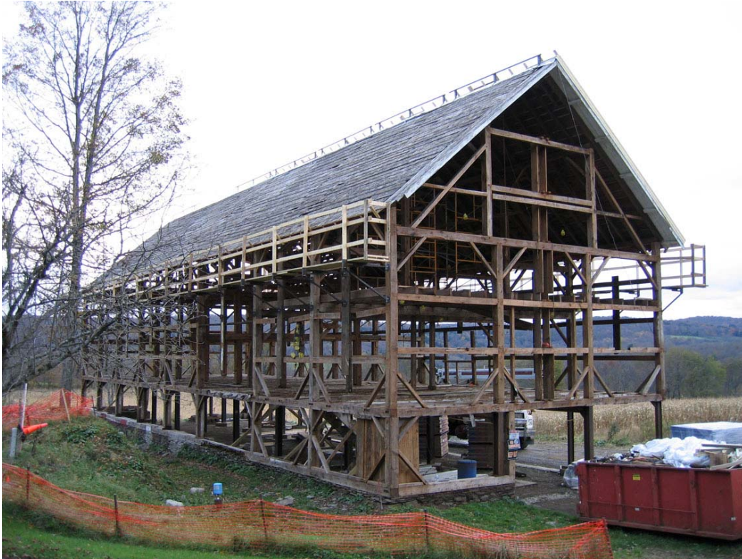
The original Golden barn getting a make-over. The scale is deceiving – note the truck parked behind.
